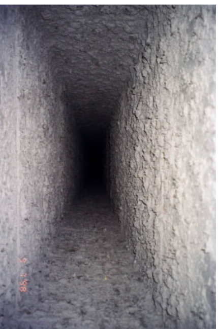
Severely Contaminated Air Duct
